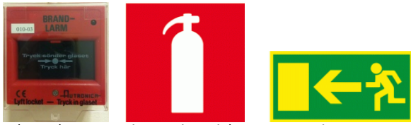
Alarm button Fire extinguisher Evacuation route
